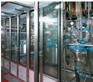
API Pilot Plant API-Pilotanlage
